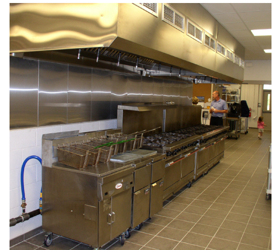
Southeastern Volunteer Emergency Services (SAVES) improved their community facility with the assistance of the Adams Electric CD Fund in 2009.
